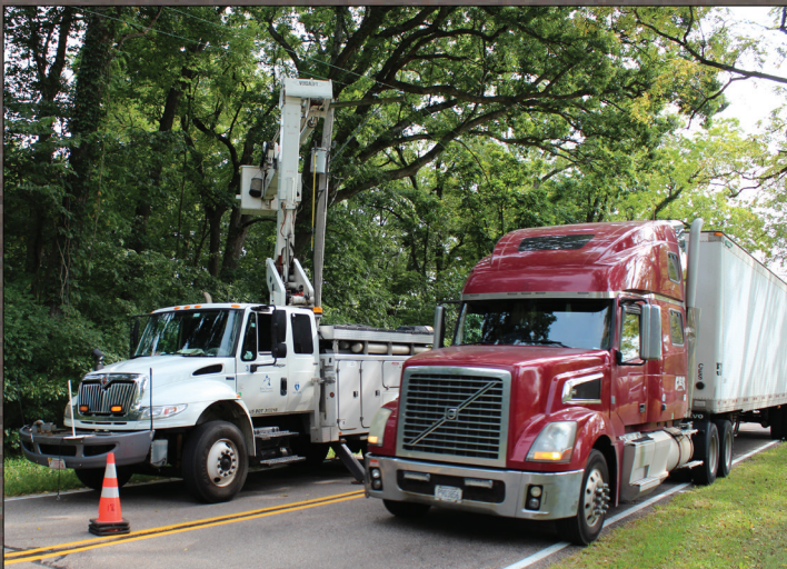
Pictured above, a Rock Energy crew works on a narrow rural road in Southern Wisconsin. In order to perform their duties, one-lane traffic was routed around the work area.
